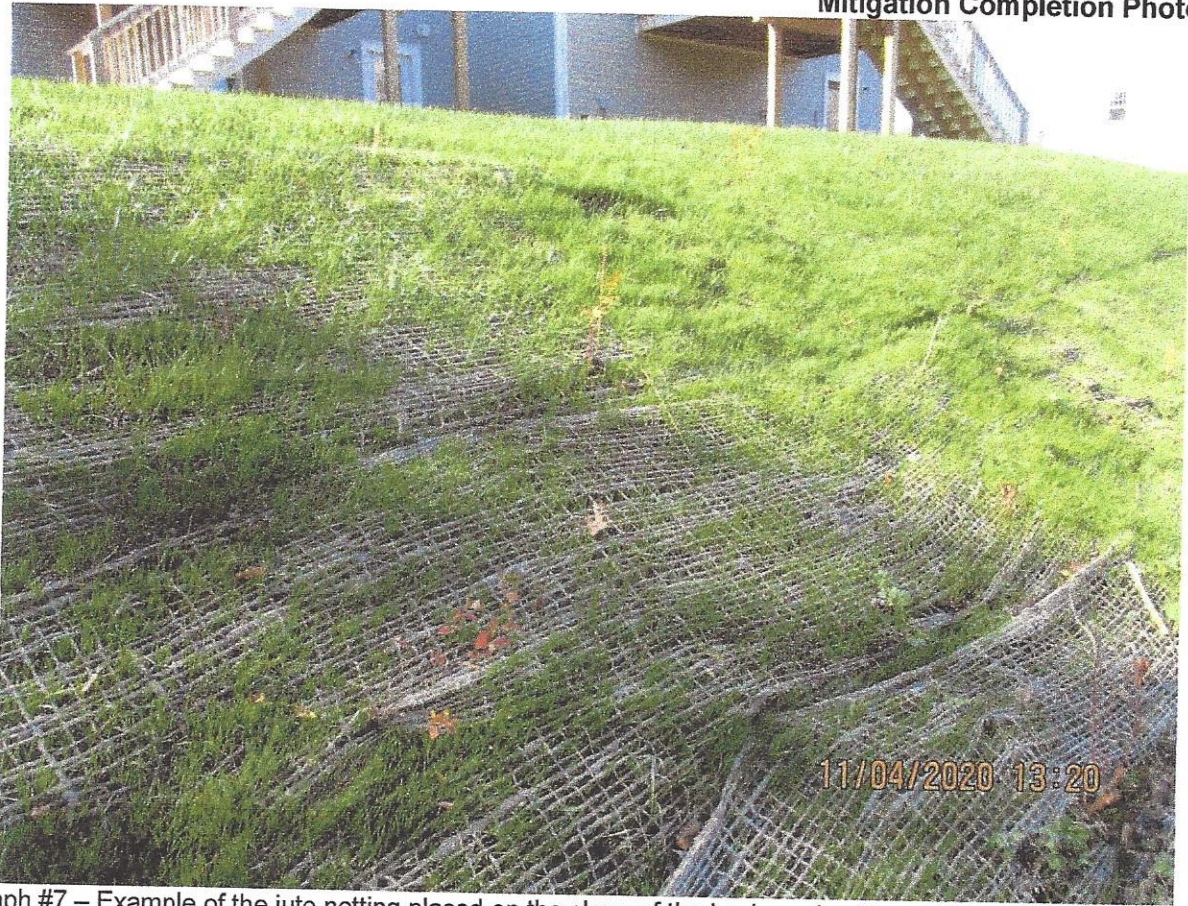
Photograph #7 – Example of the jute netting placed on the slope of the back yards. Plug plants were planted among the jute netting and then the slope was seeded.
