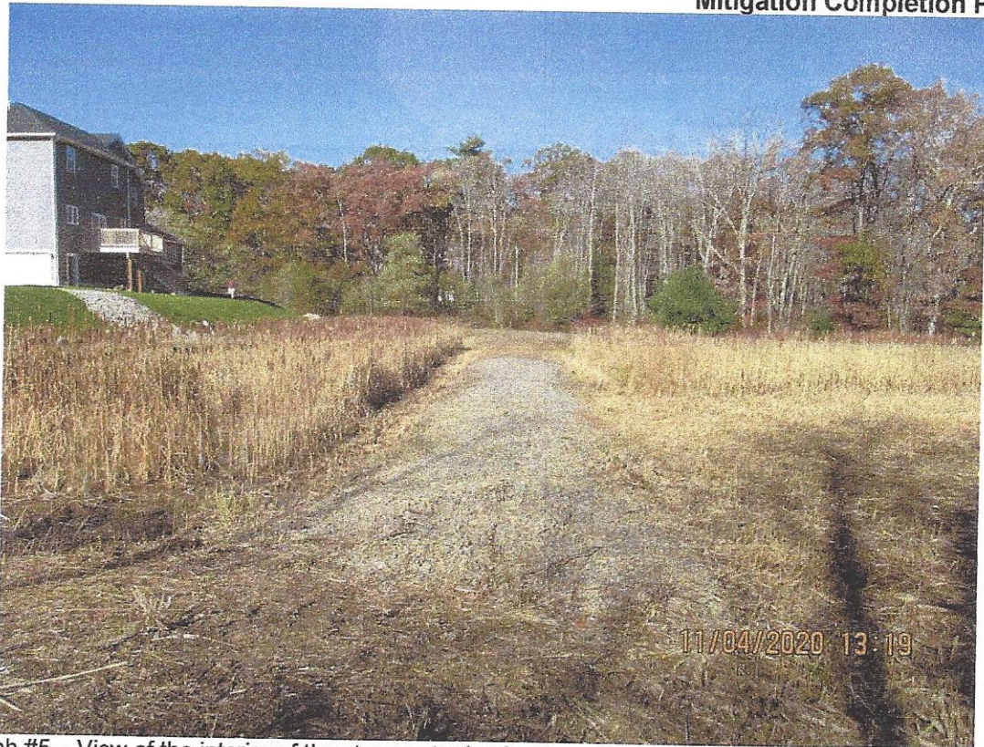
Photograph #5 – View of the interior of the stormwater basin where Phragmites was removed and the stone berm recovered.
