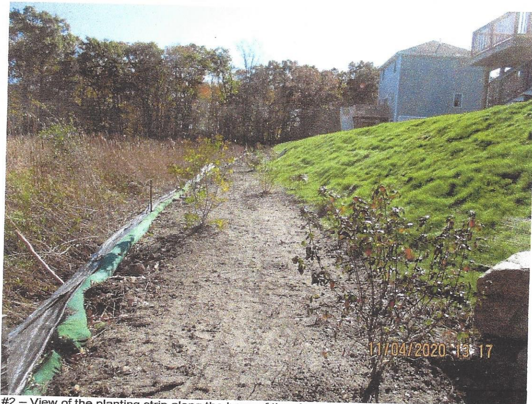
Photograph #2 - View of the planting strip along the base of the slope from the backyard area. This planting strip was loamed, planted with 30 native shrubs, and seeded with a conservation seed mix.
