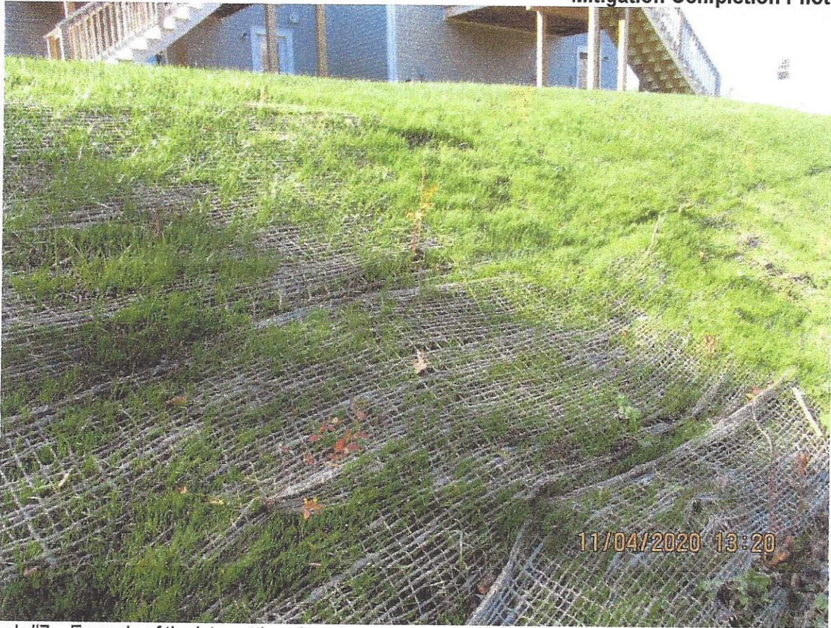
Photograph #7 – Example of the jute netting placed on the slope of the back yards. Plug plants were planted among the jute netting and then the slope was seeded.
